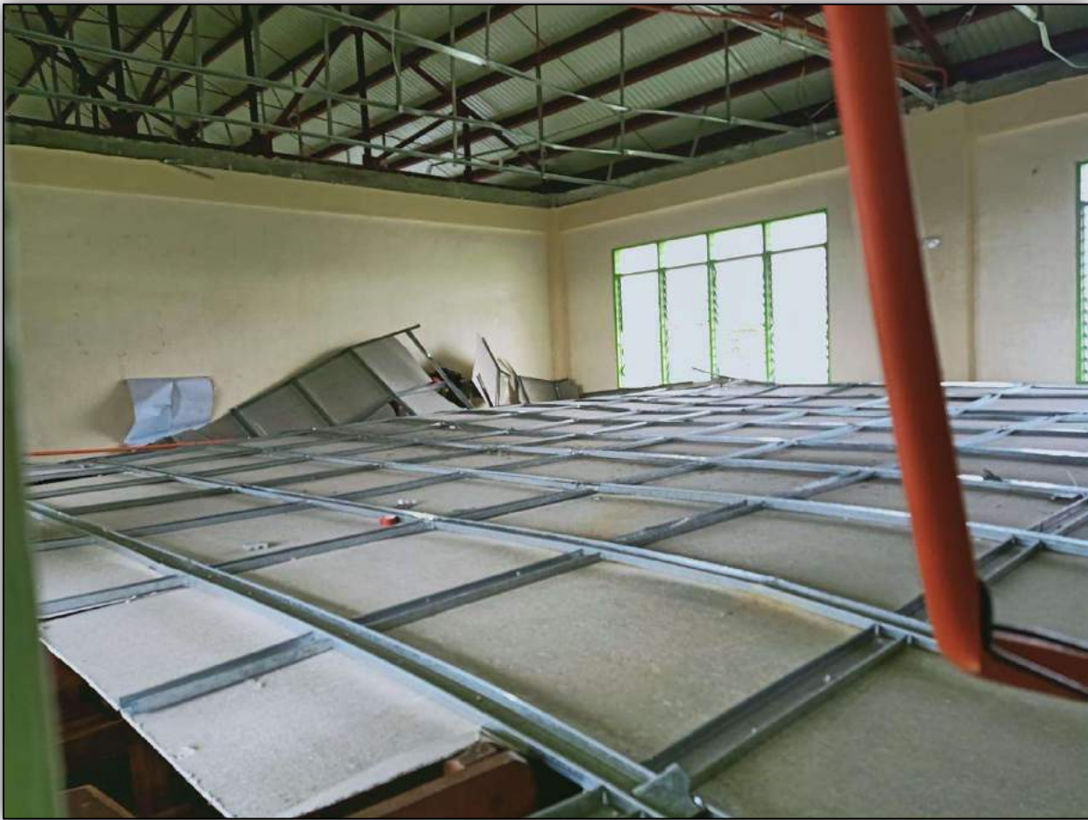
Damage to ceiling
