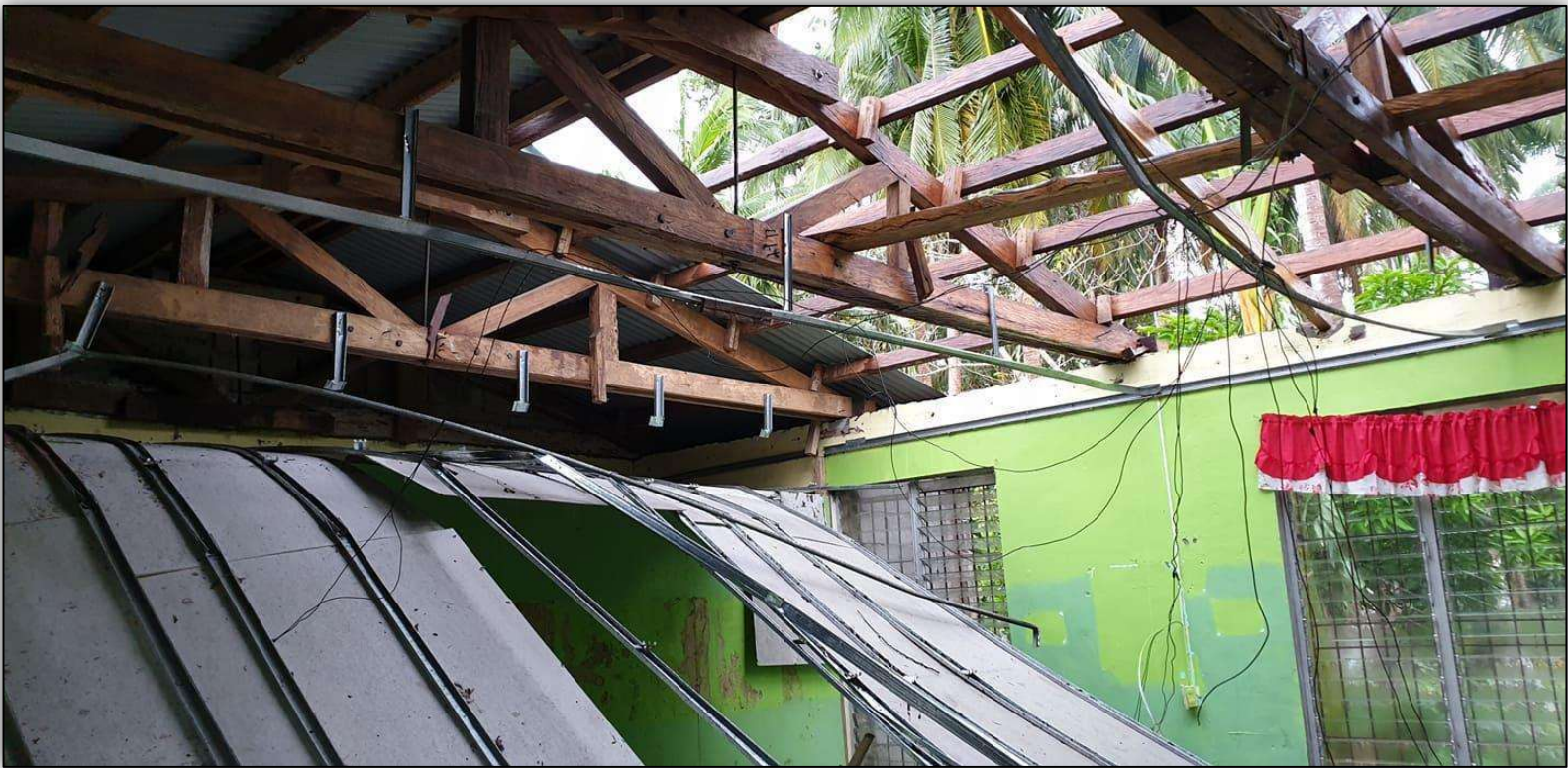
Damage to ceiling
