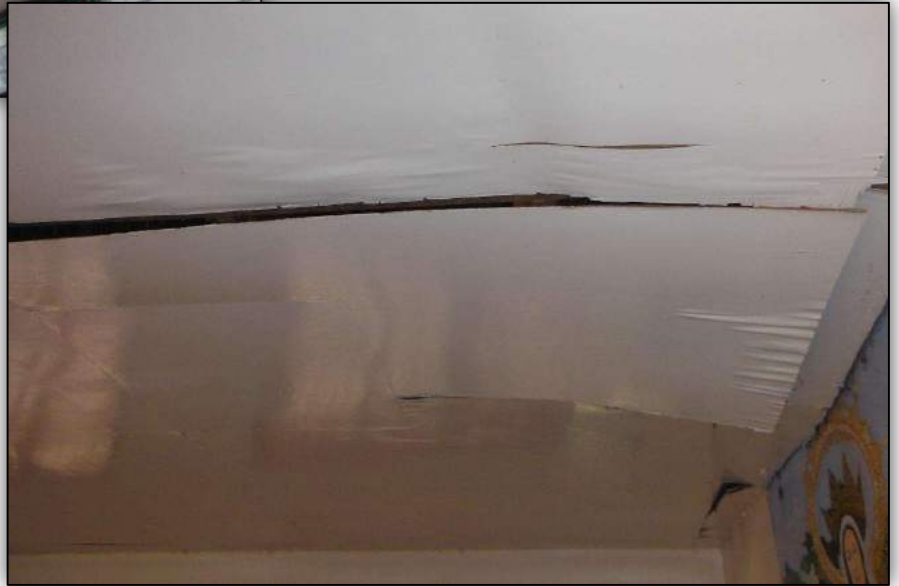
Damage to ceiling
